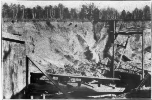
Conveyor to Screening Plant Emerging from Tunnel
